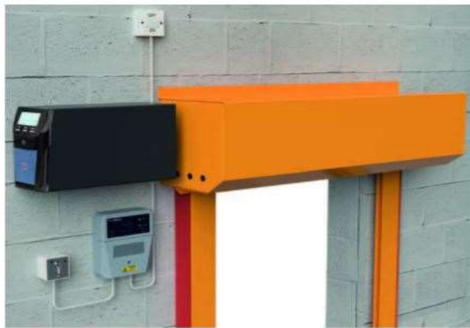
Battery Backup Unit, Control Panel & Shutter
